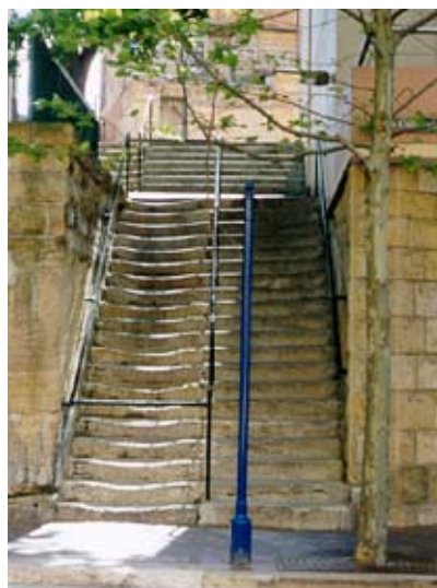
Figure 1.4 The authenticity of these Cumberland Street steps is reflected in their well worn appearance, a characteristic which has been retained by limiting the installation of new operational treads, and access, to the right-hand side.
