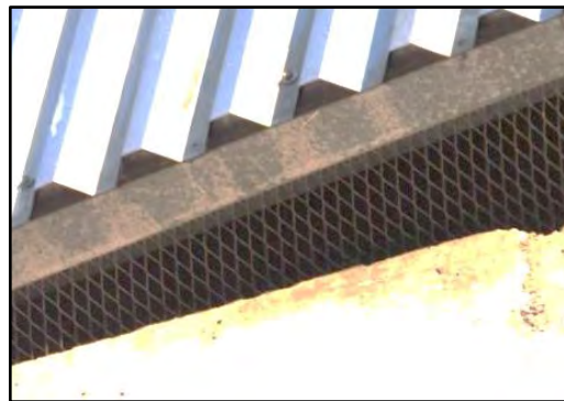
Photo 5 - Large mesh openings on reservoir
