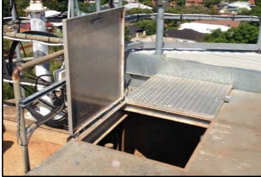
Photo 1 - Service reservoir hatch left open
