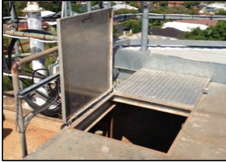
Photo 1 - Service reservoir hatch left open
