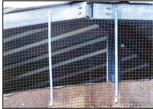
Photo 4 – Deficient reservoir roof design
