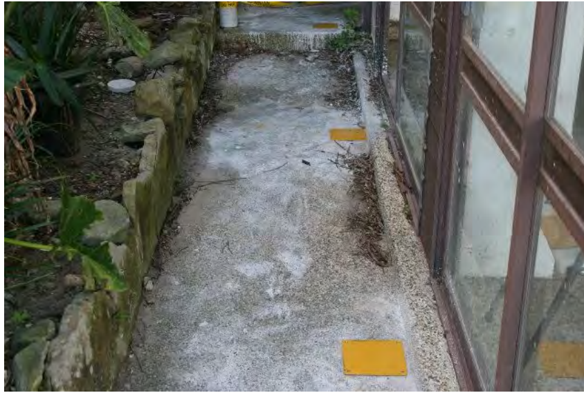
Photo 5. Capped bore holes in pathway beside the building
