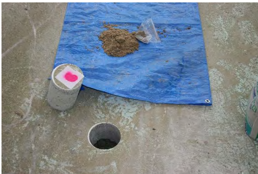
Photo 4. Bore hole through concrete floor slab, and soil sample inside the building
