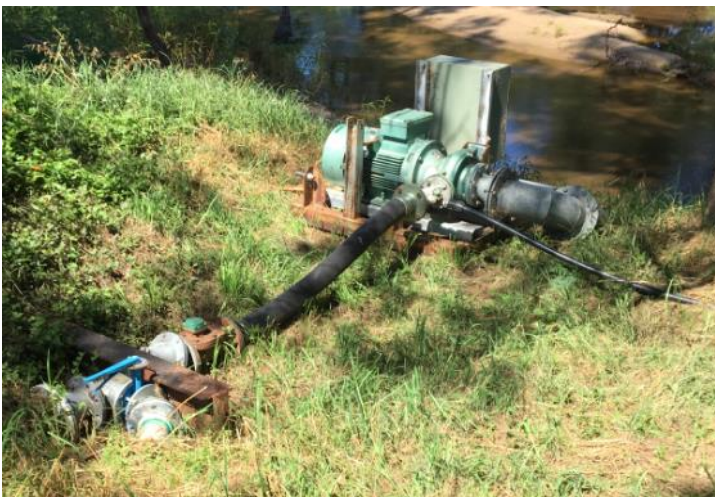
Figure 4. Portable pump secured in position on a typical riverbank
