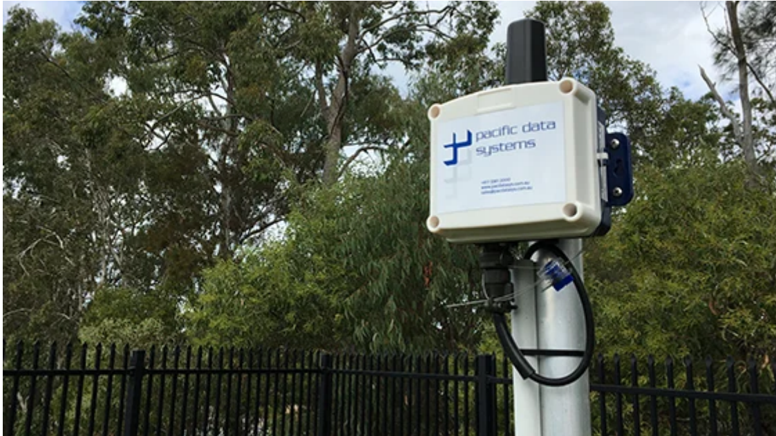
YDOC Local intelligence device. Credit: Pacific Data Systems Australia.
