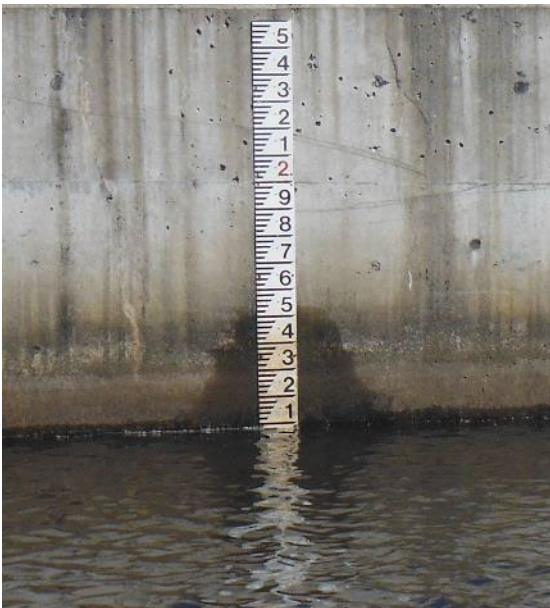
Figure 1. Depth Gauge Board installed on a concrete storage wall
