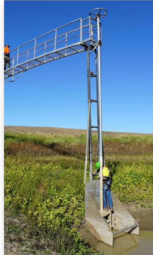
Submersible Pressure Sensor – affixed to the deepest point of the storage
