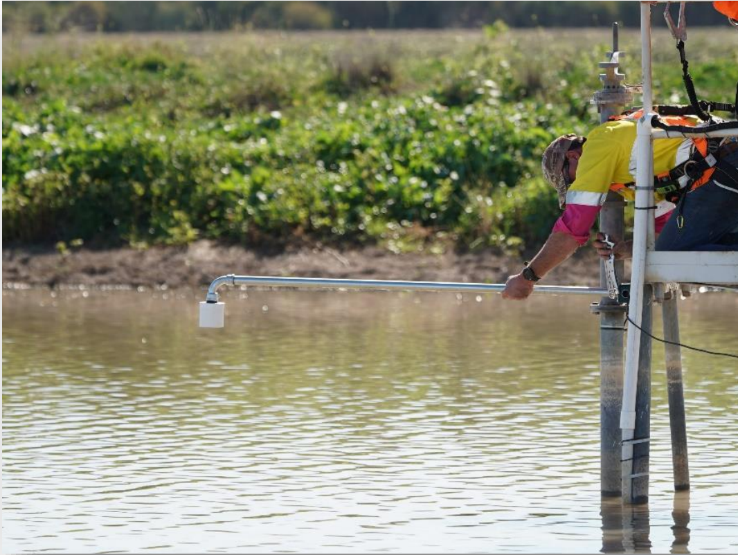
Radar Sensor – measures water level using radar from above (catwalk)
